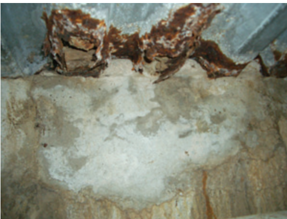
Figure 1-4 Corrosion of galvanized fluted steel floor deck. The floor is at grade level. The source of the water is rainwater seepage.
