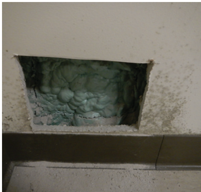
Figure 4-1 Interior Wall Showing Water Damage and Mold
