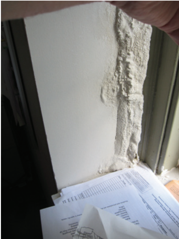
Figure 1-10 Further rain damage to interior plaster. At another location on an office window in the building shown in Figure 1-8, rain seepage turns gypsum board joint compound to a fluid, causing the gypsum to bubble and lift.
