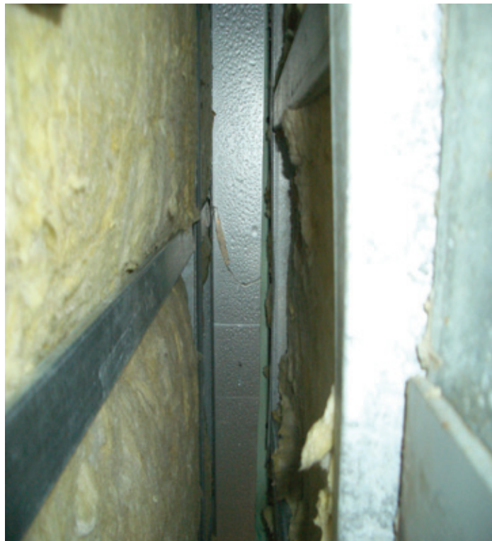
Figure 1-20 Condensation on Uninsulated Metal Framing in a Cold Climate
