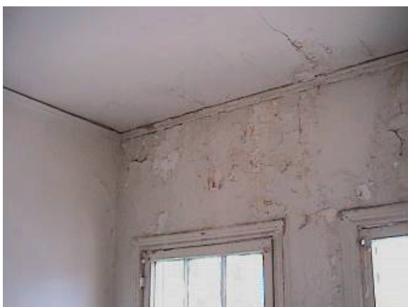
Figure 1-8 Rainwater leaks in a rooftop parapet wall result in damaged plaster and peeling paint. Rainwater is drawn into this brick assembly by capillary action, and the moisture is aided in its downward migration by gravity. The peeling paint contains lead and results in an environmental hazard as well as physical damage to the plaster.
