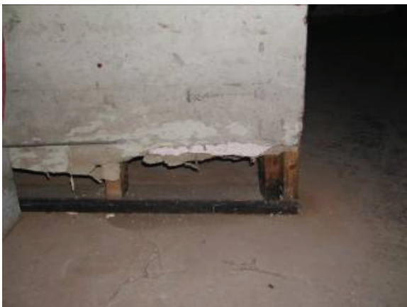
Figure 1-11 Gypsum board on the lower edge of a basement wall dissolved by seasonal flood waters. The water table is just below the basement floor during dry weather and rises several inches above the floor during heavy spring rains.
